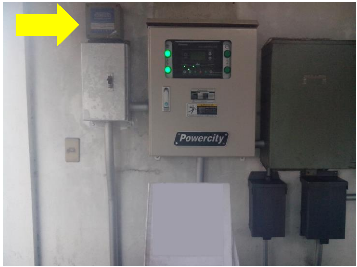
Figure 3 – An example of SPD at Utility Feed Disconnect
